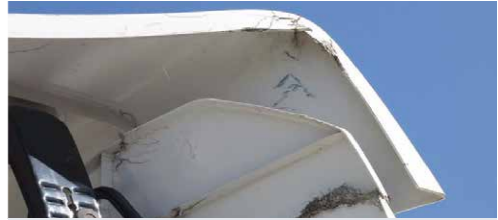
✗ Severe formation of cracks
