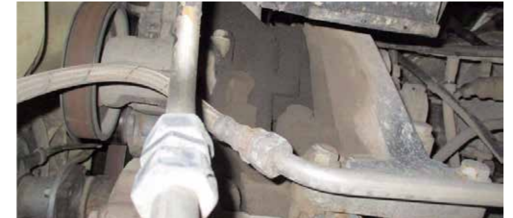
✗ Oil loss at engine
