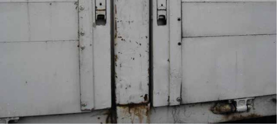
✓ Minor wear on the side wall
